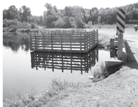
Photo: One of two new floating docks installed alongside the bridge over Black Creek in Espanola
