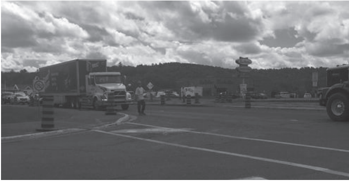
Photo: Phase three of the resurfacing of Highway Six in the Town of Espanola includes the installation of lights. Espanola council approved the third phase of the connecting link project from MacDonalds to Second Avenue on Centre Street in late June at a cost of just over $6-million dollars accepting the bid from Garson Pipe Incorporated. Photo by Rosalind Russell
